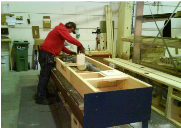
Fig 18. The BoKlok Service Wall being manufactured off site in factory controlled conditions. Each service wall uses continuous pipework to primary locations for fittings, such as basins. This ensures that only one connection is used per fitting minimising the potential for leaks within the dwelling(s).
